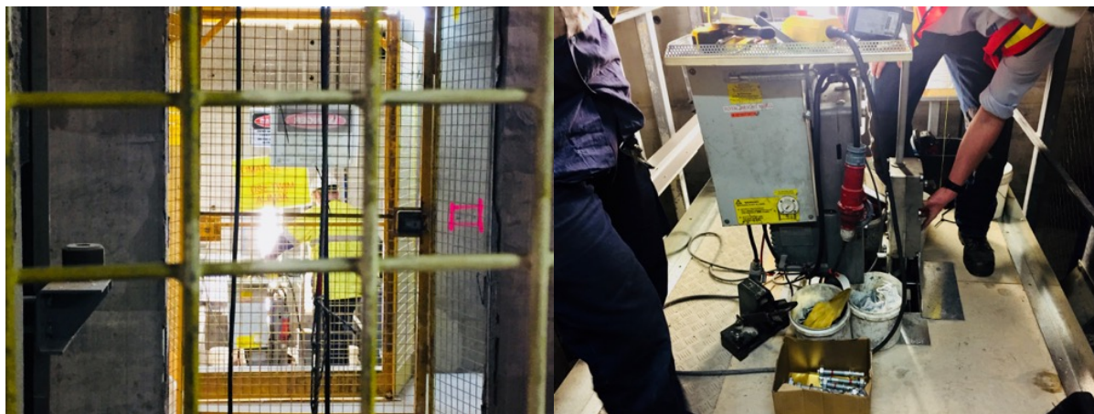
Figures 6.5 and 6.6: Assembling the “jump lift” on the construction site of a residential high-rise tower, Melbourne CBD, October 2017. Photo: L. Dorignon.
